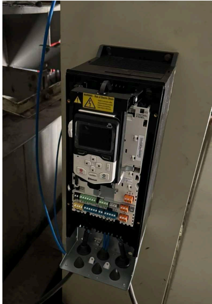
Figure 3.1 Inverter installation at electrical cabinet
