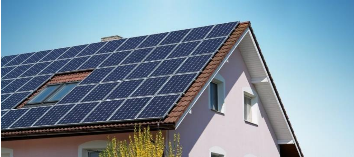
Figure 10. Rooftop PV system on a gable-roofed house
