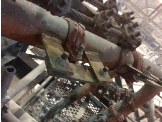
Figure 1.6. Current prevention of lime coupling failure. Welded brackets and safety truss.
