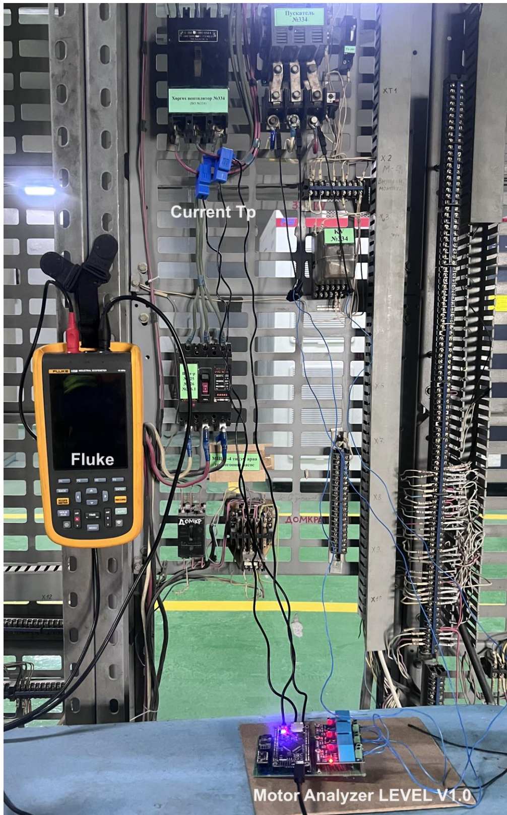
Figure 26. Measurement by the data acquisition system in the field
