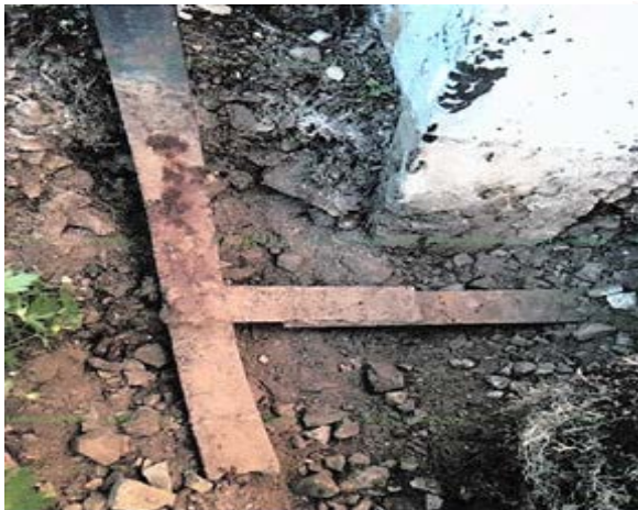
Figure-17. Podiem-3: 110/6kV substation 1st transformer deep neutral grounding
