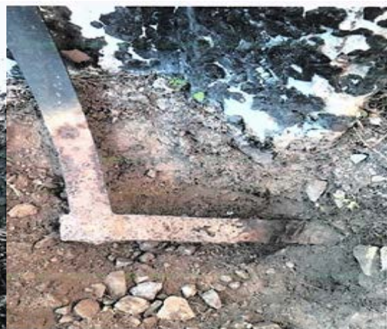
Figure-18. Podiem-3: 110/6kV substation grounding grid outer belt conductor
