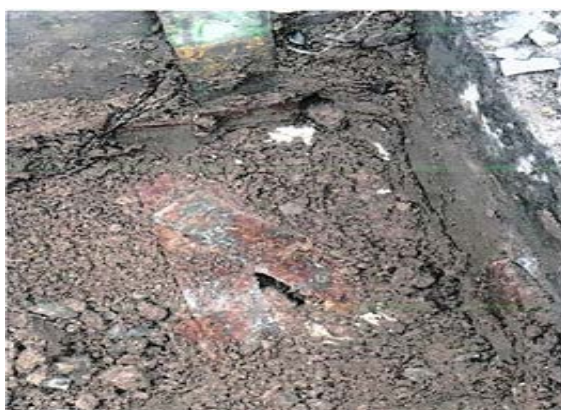
Figure-19. TSRP-1 Zest TETS 110/6/6kV substations' C phase belt input grounding
