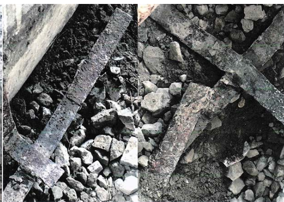
Figure-20. RP-1. 110/6/6kV substation's 2nd transformers deep grounding
