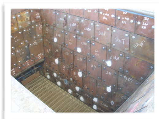
Figure 24: Liners inside a chute
