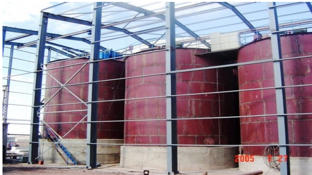
Figure 6 Leaching and adsorption tanks
