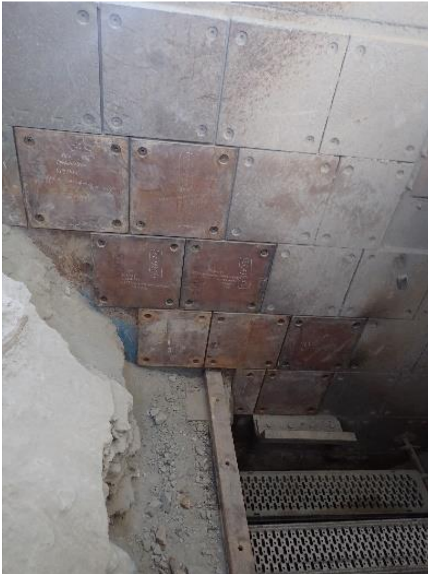
Figure 30. OT Discharge chute CVB-001 linear
