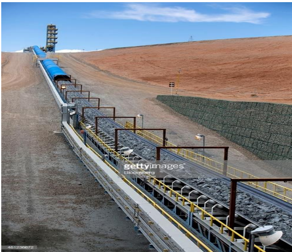
Figure 28. OT Primary Crusher conveyor
