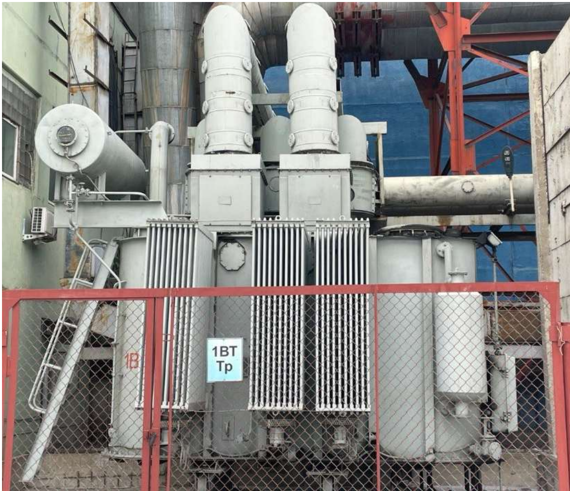
Figure 3. External view of Auxiliary Transformer 2BT
