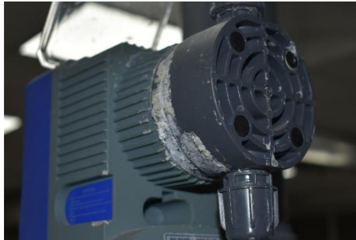
Figure 20: The peristaltic pump failure and sulphuric acid drop from pump
